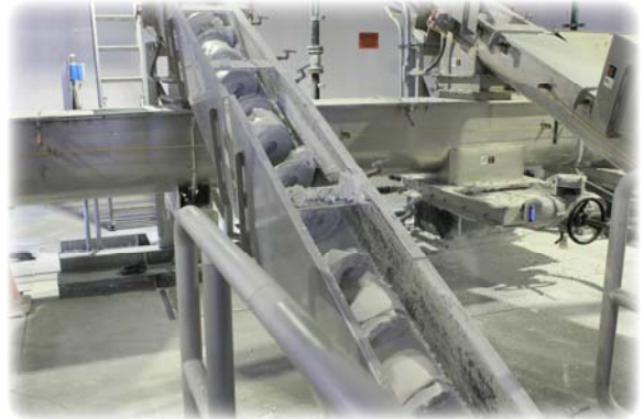
Extracted Salt at the Chino Desalter Authority II Facility
